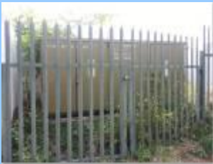
3Phase 200KVA transformer
