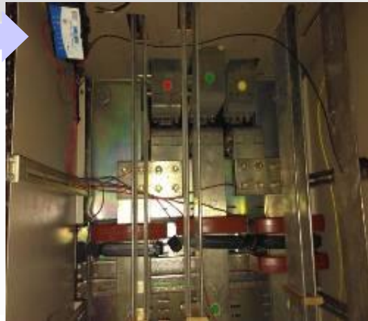
Main Power Cabinet
